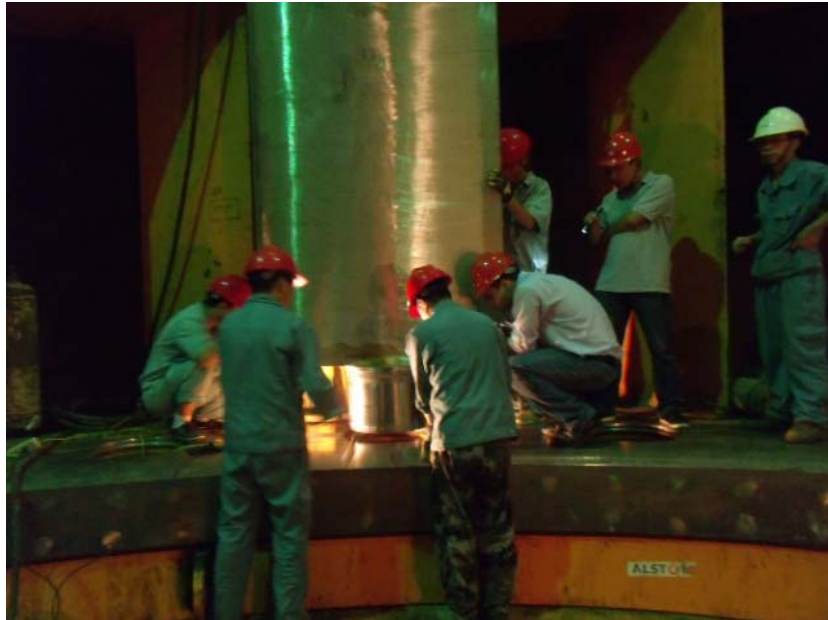
GGB Hydro Group's Edward Chen (holding flashlight) and William Barreto (kneeling right) assist in the assembly of the first wicket gate for China's new Xiangjiaba hydropower plant.
